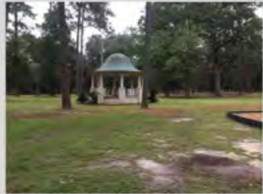
Current condition of the gazebo is not good. It seems to be failing structurally, and is also quite small.
